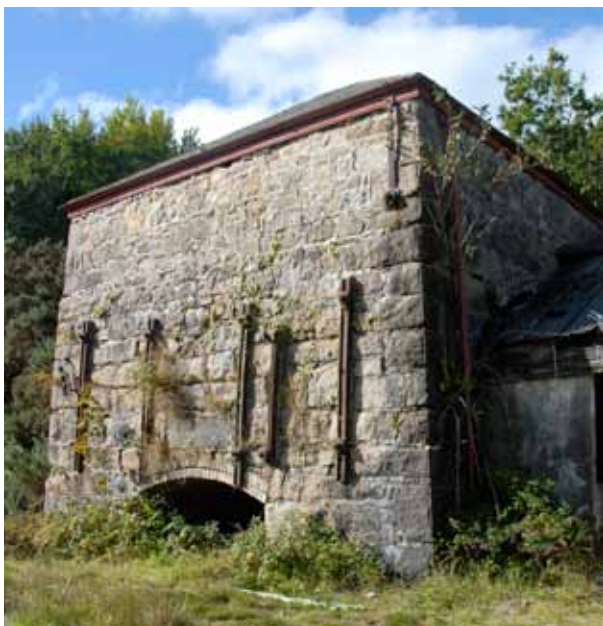
Above: The Tolgus Calciner near Redruth, the most complete example of this rare ore dressing structure
